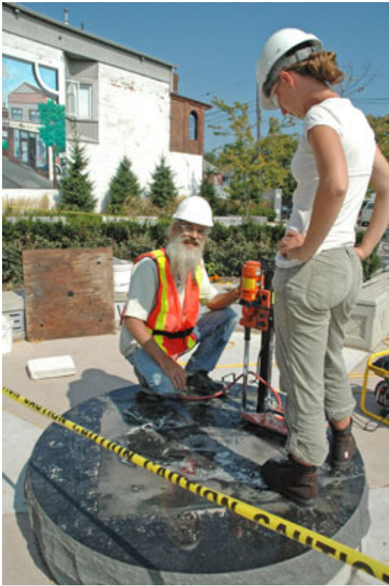
Left: Daniel with assistant. Beginning the installation a week before the unveiling.
